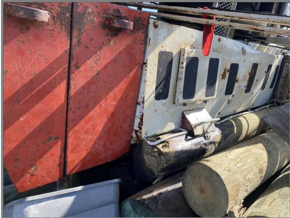
View of damages to upper catwalk
