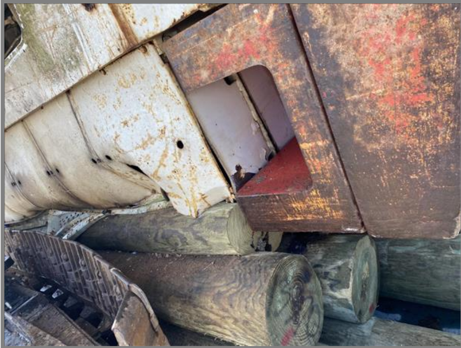
View of structural damages to tunnel
