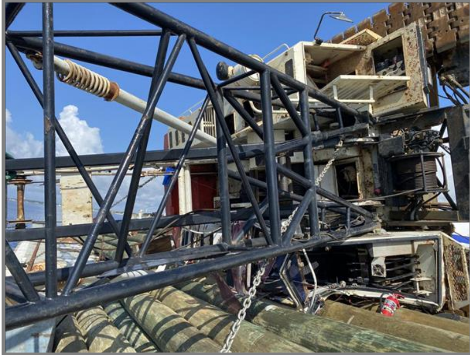
Boom base damages
