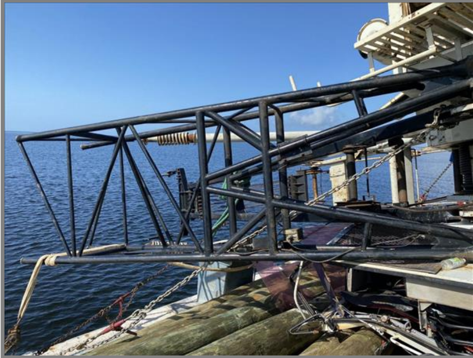
Damaged base section of boom
